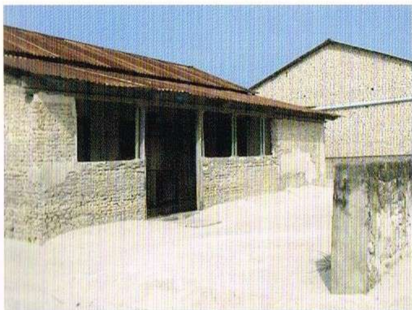
Image 6: Chipped coral masonry construction
